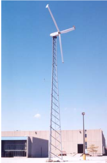
Enertech 40 kW in Urban Locale
